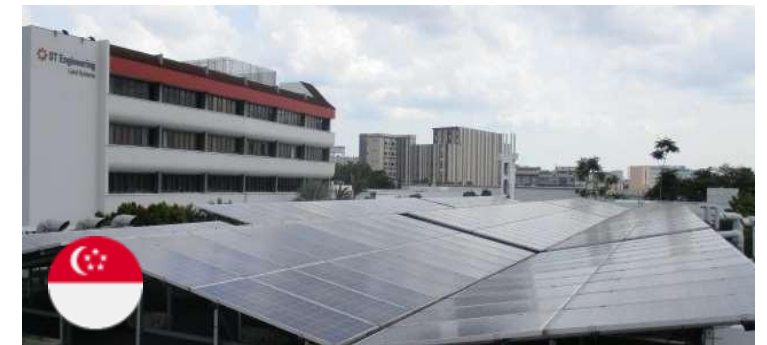
Location: Jurong, Singapore Capacity: 120.9 kWp Contract: 25 years PPA with ST Kinetics Ltd.
