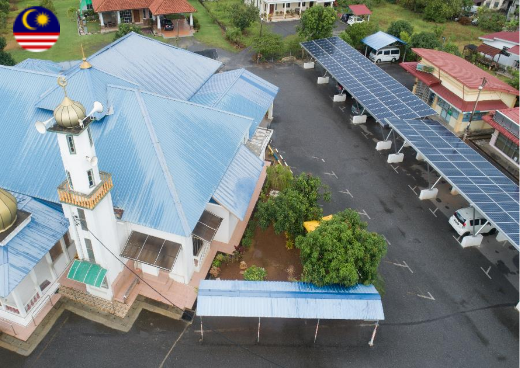
Location: Perlis, Malaysia Capacity: 47.85 kWp
