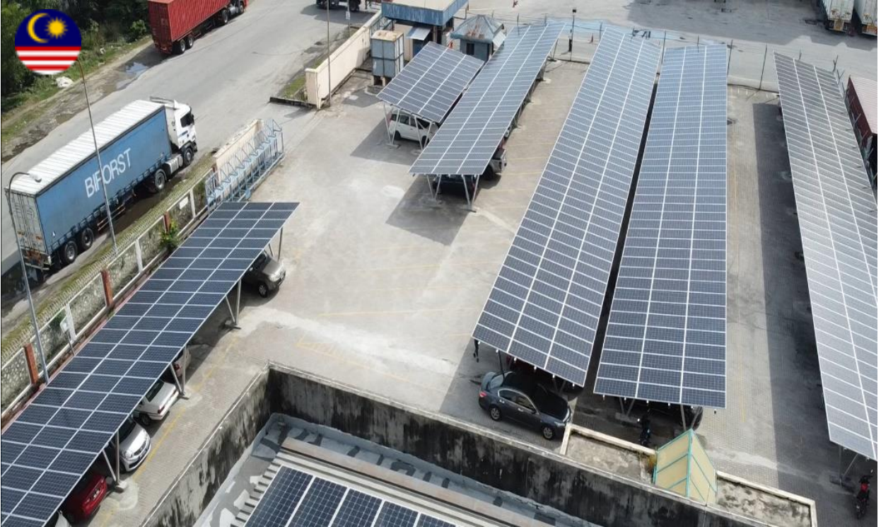
Location: Selangor, Malaysia Capacity: 8.6 MWp
